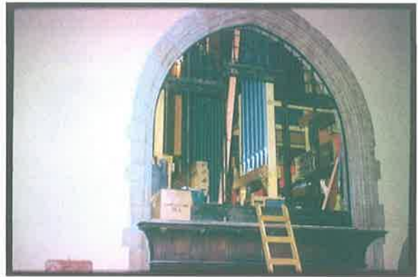
Schlicker organ installed in organ chamber (38)
