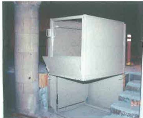
as was an ADA-compliant elevator (96)
