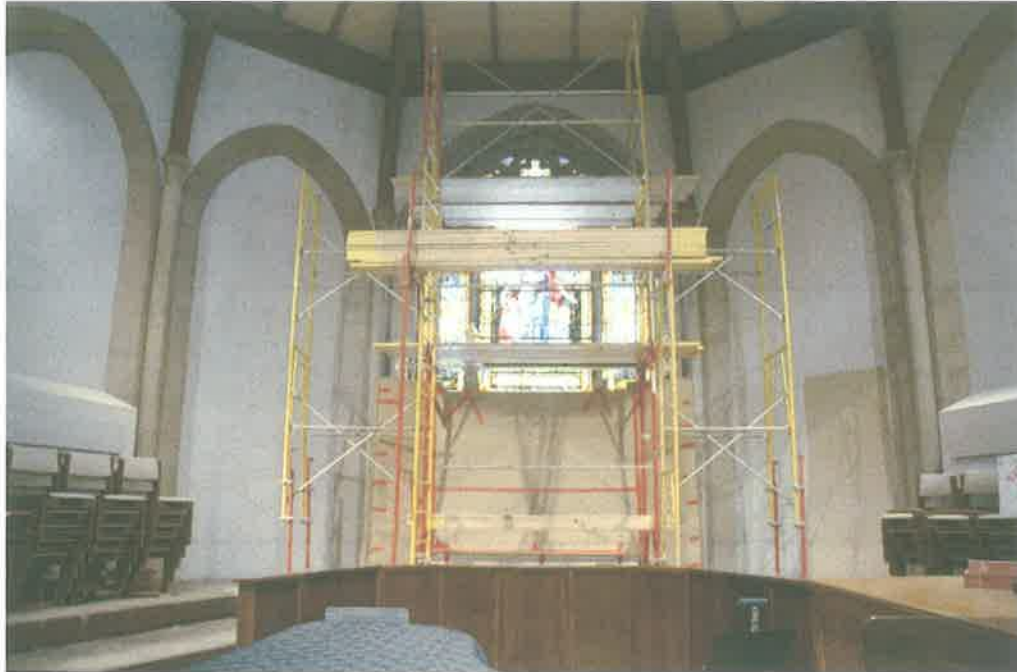
On January 2, 2007, scaffolding was put in place in the inside and outside of the church. On January 3 and 4, the three windows were removed and replaced by plywood. The windows were taken to the Judson Studios in Highland Park for restoration. (209)
