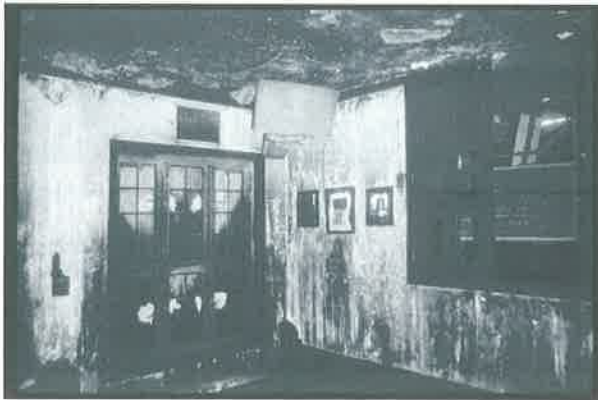
Fire damage to the Guild Room (43)
